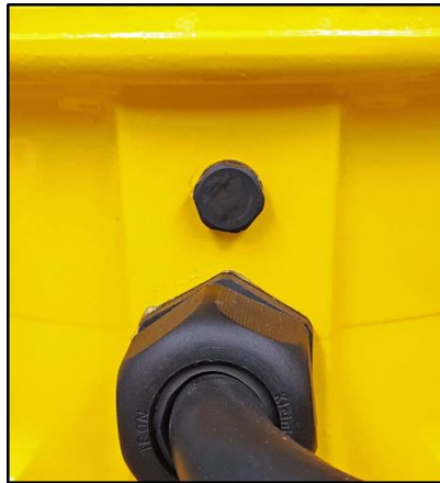
Beacon PFB-37003 with PL10961-M12-HF Vent Installed above the cable entry gland
